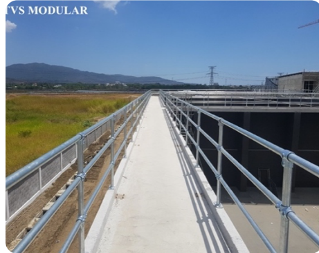
WATER TREATMENT HANDRAIL
